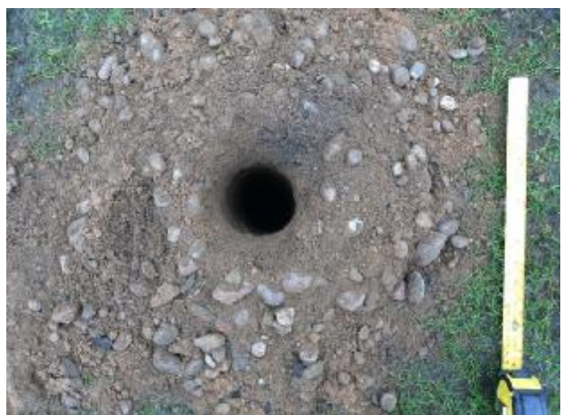
Figure 6: A friable and free draining medium is employed at depth in the construction but the compaction of the materials above, and a lack of formal pipe-drainage, is rendering the surface unplayable.
